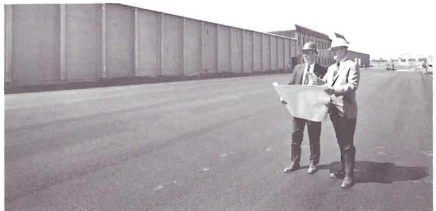
Bill Young, Assistant Manager of Engineering, and Lee McClary stepped out of the construction area for a moment to take a look at the new plant from one end to the other – a very long look.
