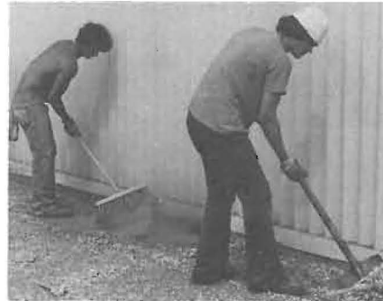
Workmen at left begin the job of roof restoration, while (below) the front roadway gets a face lifting.
