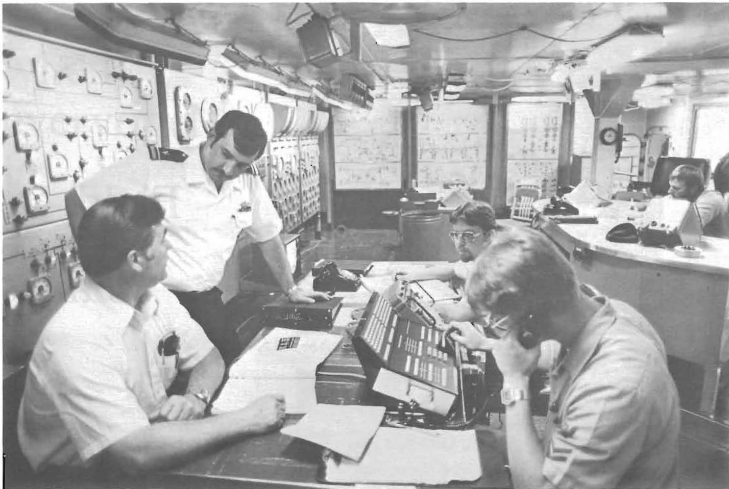
SHIPPING OUT WITH THE FLEET. Walt Knapp, (seated left) Western Electric supervisor at the Guilford Center, briefs Electrical Officer Lt. (jg) Rene Fry and crew on the performance of the Dimension® 2000 Private Branch Exchange. The PBX was recently installed aboard the aircraft carrier John F. Kennedy and will handle all internal communications. Manufactured at Western's Denver, Colo. plant, this Dimension PBX is the first electronic PBX on a tactical ship.
