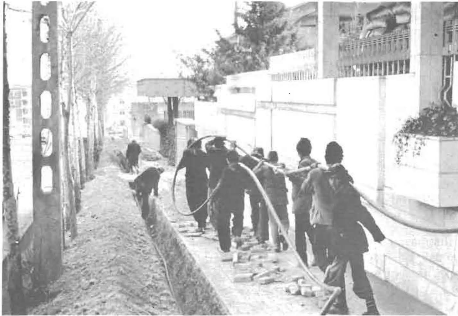
Before the Iranian Revolution, American Bell Inc. was involved in developing an advanced telephone system in that nation including the installation of underground cable.
