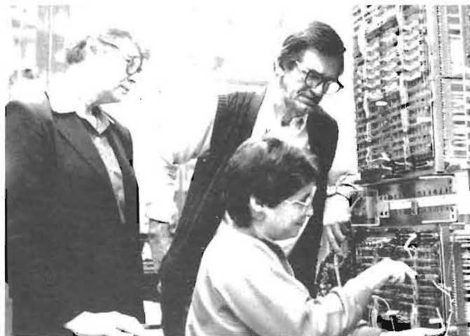
Faye Knipe and Don Nadeau watch for proper insertion of a cable wire receptacle onto a blade by wireperson Chris Tuccolo.
