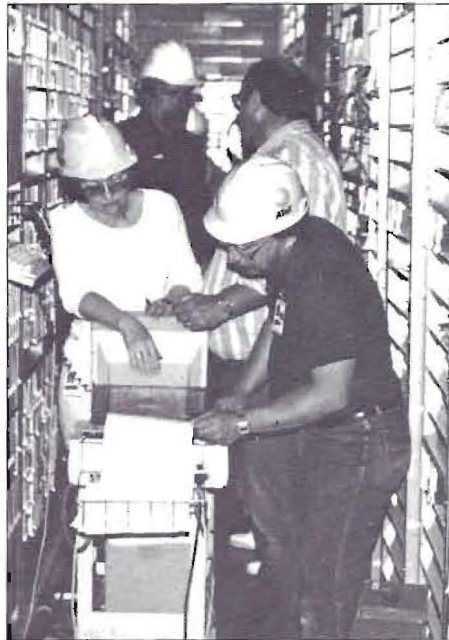
Sandy Krause, left, senior engineer, performs installation test on one of the newly installed D5 systems.
