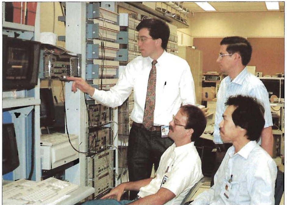
TIM HAAS of the DACS Installation and Technical Support department reviews DACS II operation with RTAC's Eric Puetz, Pat Dulatt, and Jackson Lew.
